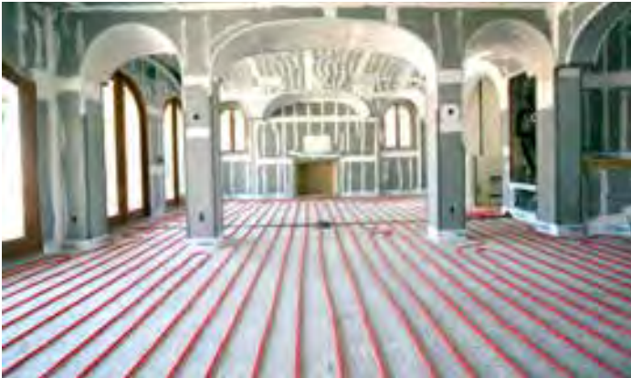
Infloor residential hydronic heating system.
